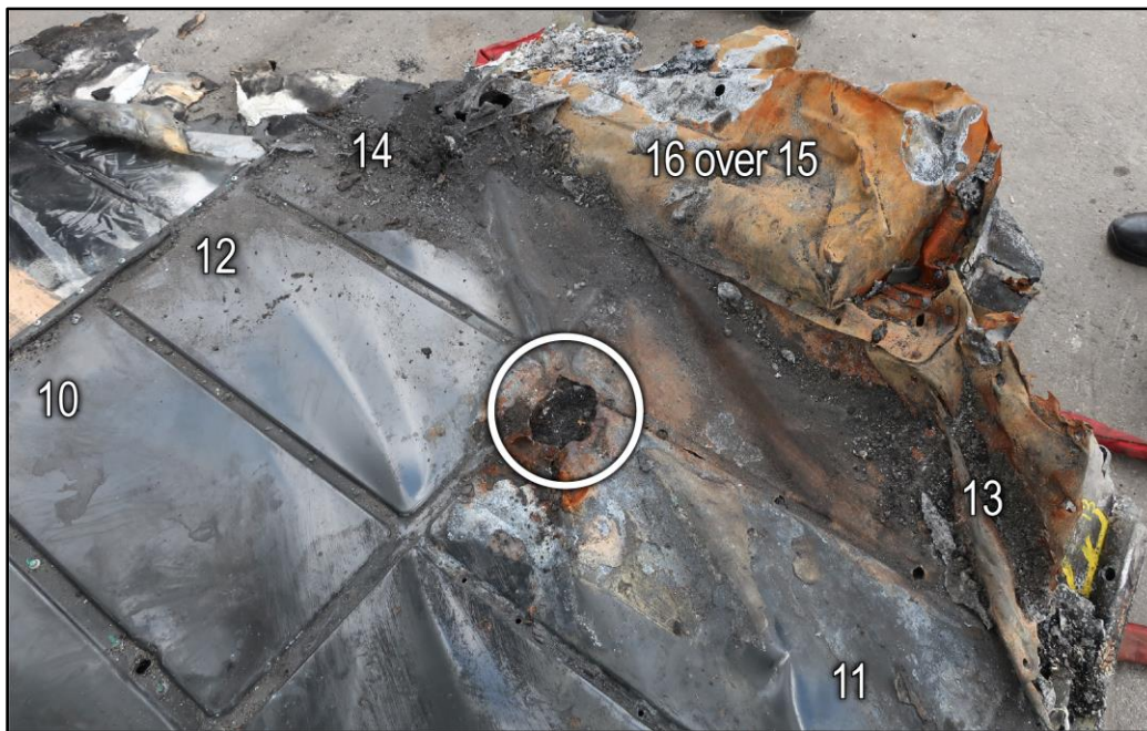
Figure 12. Top surface of forward part of battery case showing damage to front and hole melted through steel cover (circled), with modules numbered.
