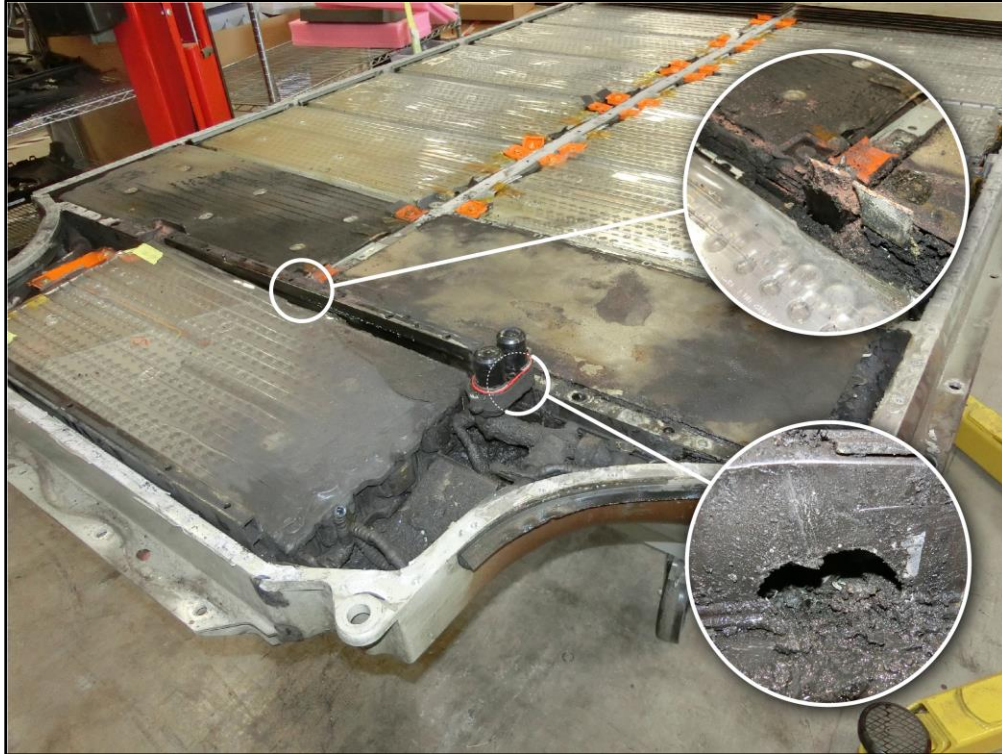
Figure 15. Battery pack with top cover removed to show location of holes in battery case and insets showing closeups of damaged areas.
